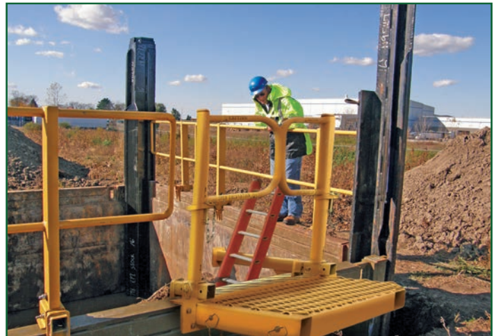
Guard Rail with Ladder Platform
